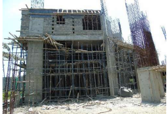
-Column & beam steel work underway. -Blockwork in parts of 3 rd floor done.
