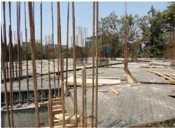
Column rebar and formwork for slab concreting on parts of ground floor underway.
